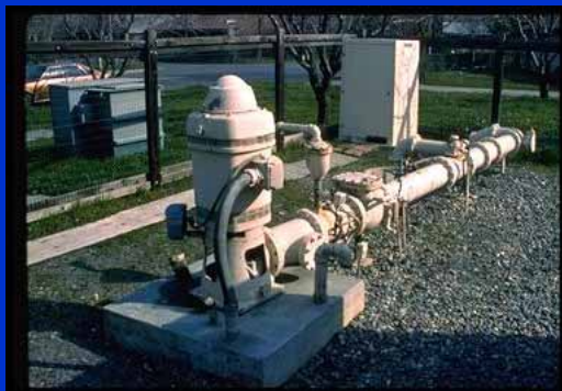
Public Supply Well at a Water Treatment Plant
